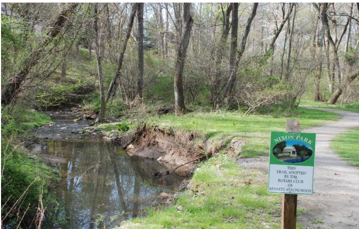
Eroded stream bank threatens trails
