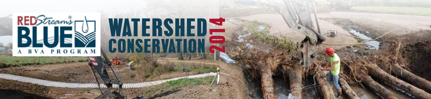
Contractor installs a cross vane below a new livestock crossing on the Upper West Branch in Honey Brook.
